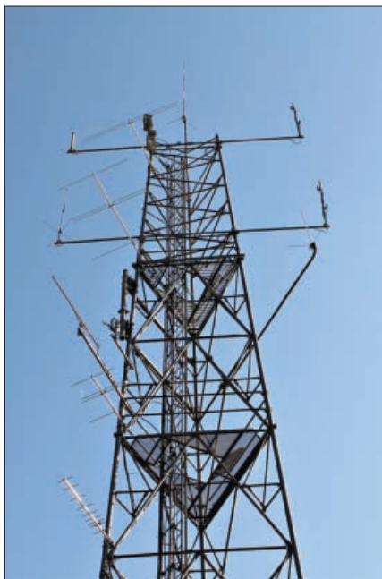
The mast carrying the GB3MCB beacon antennas on Hensbarrow Downs in Cornwall.
